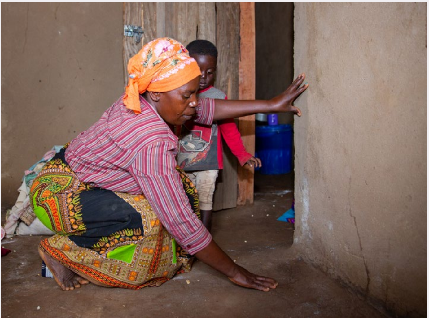
Bertha, mother of four and savings group member, feels the damp ground of the room that used to be her bedroom before her home was flooded during Cyclone Freddy in Malawi.
